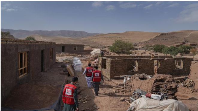
1st October 2024: Rebuilding after the devastating earthquake - Afghan Red Crescent Society and IFRC workers constructing transitional shelters in Zinda Jan and Gulran districts. (Photo: ARCS)
