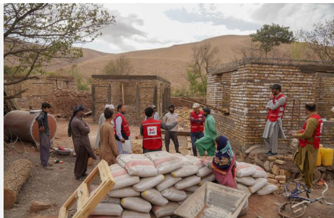
ARCS and IFRC staff jointly monitoring the construction progress of earthquake relief shelters in Zinda Jan district, Herat Province on 1 October 2024 (Photo: IFRC)
